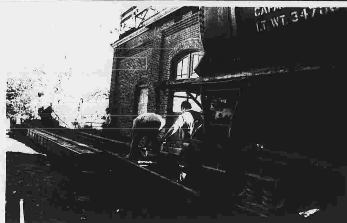
Workers prepare to move a railroad tank car, once part of the historic South Manchester Railroad, onto a flatbed truck this morning. The 17-ton car was discovered in a shed behind the Clocktower Mill building on Elm Street
